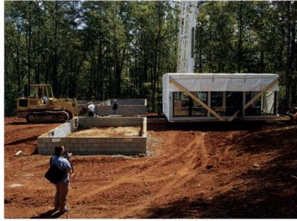
Clockwise from far left: Trucks make their way up the newly created Beech Hill Road with the modules; homeowner Nathan Wieler documents the process; modules are lowered onto the foundation.
