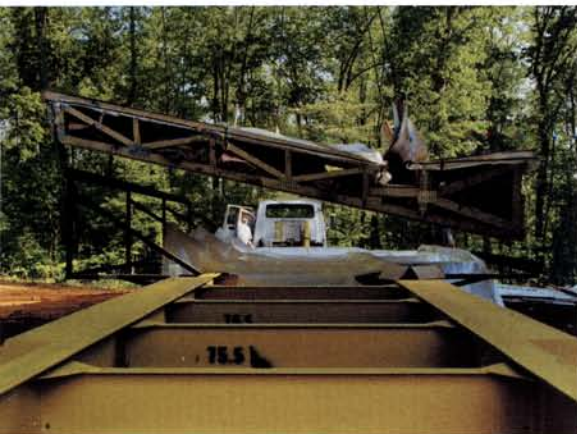
At left and below: The crane operator deftly installs the roof modules. Not shown are workmen, architects, and clients holding their collective breath.
